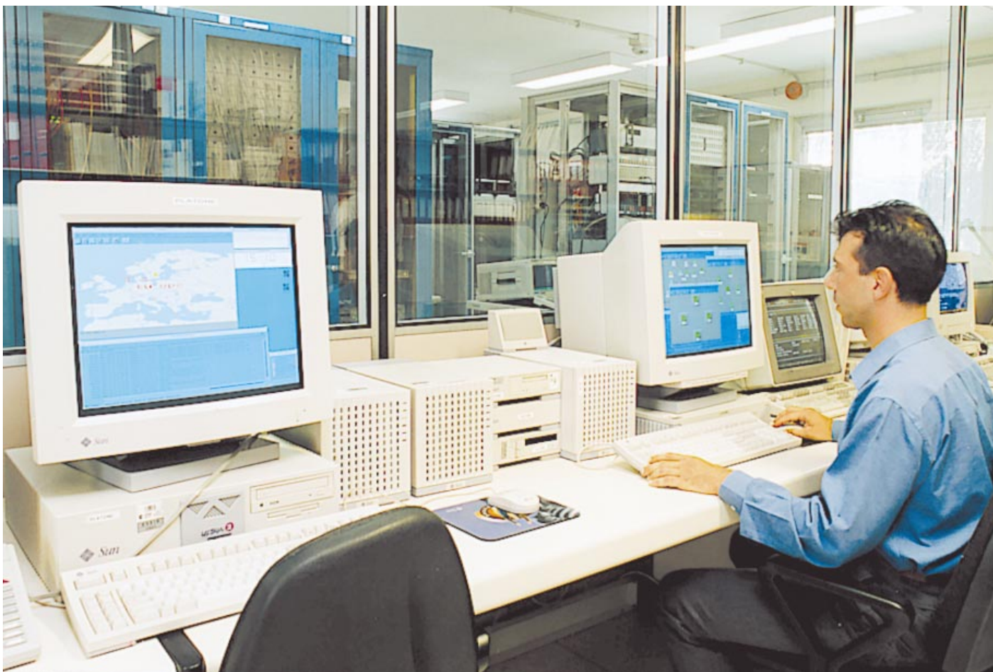
Figure 5. The ESACOM Network Control Room
