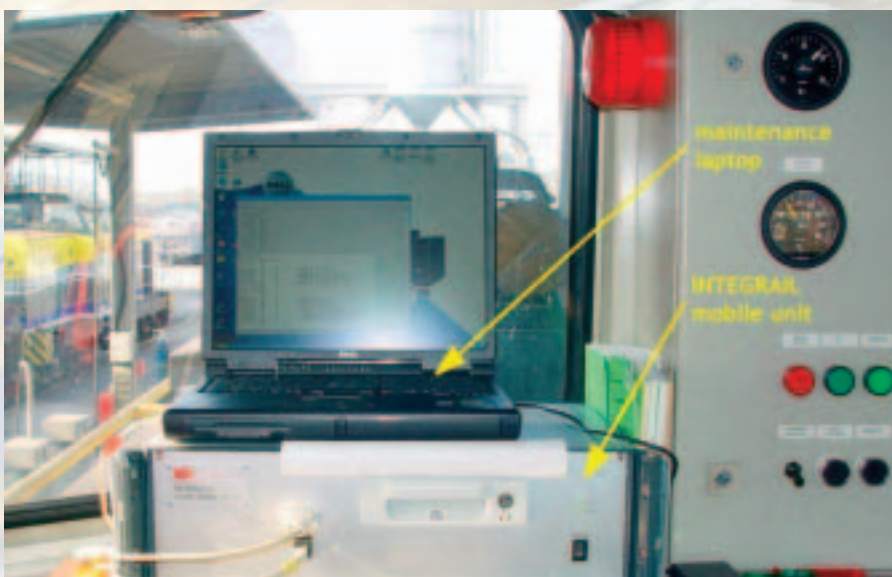
The INTEGRAIL unit installed in a locomotive for test purposes (Courtesy of Bombardier GmbH)
