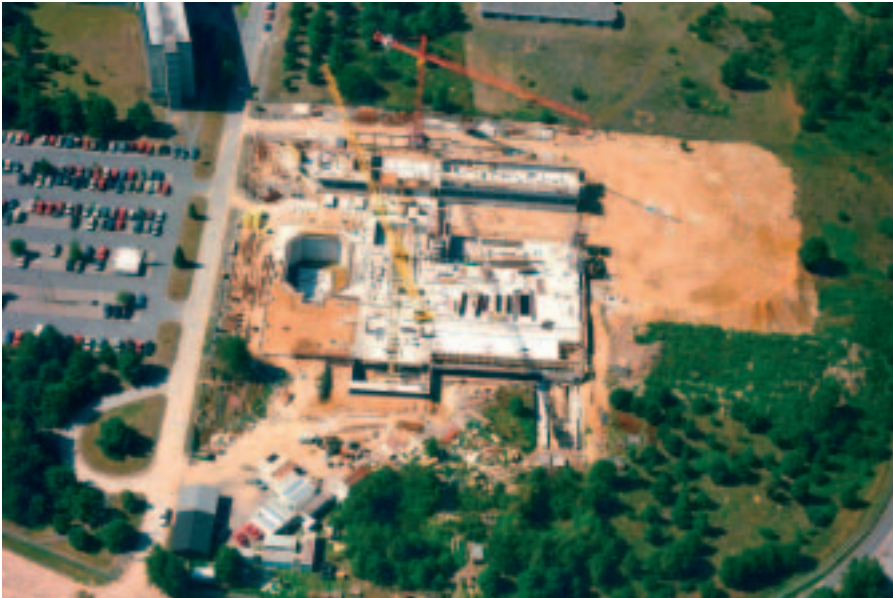
Construction of DLR's CTC building, with its Neutral Buoyancy Facility, in August 1991
