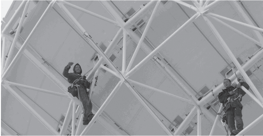
The supporting structure of the Cebreros antenna
