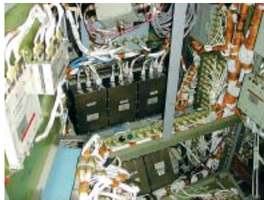
The two FTCs installed in Zvezda are literally black boxes.
